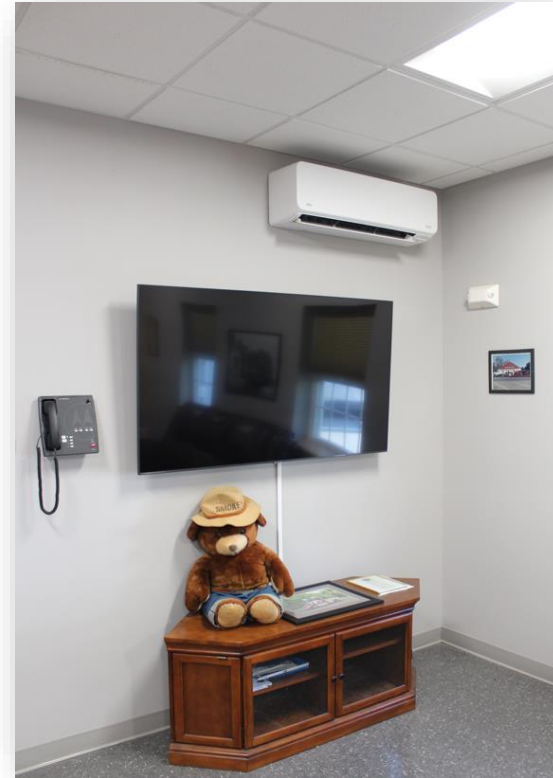
Heat Pump in Norridgewock Fire Dept.
